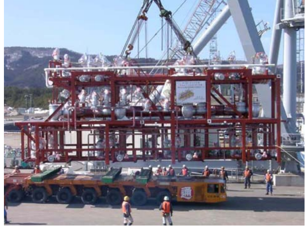
Figure 10. Piping Module (Source: Toshiba, 2009)
